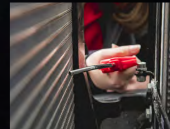
Plenty of room to access radiator for cleaning.
